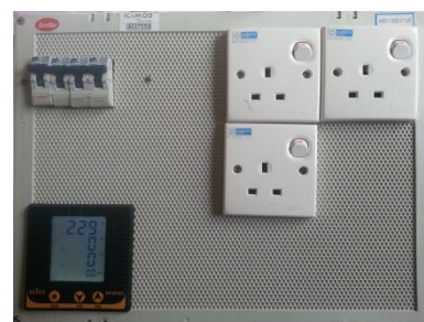
Fig. 1 Digital energy meter
